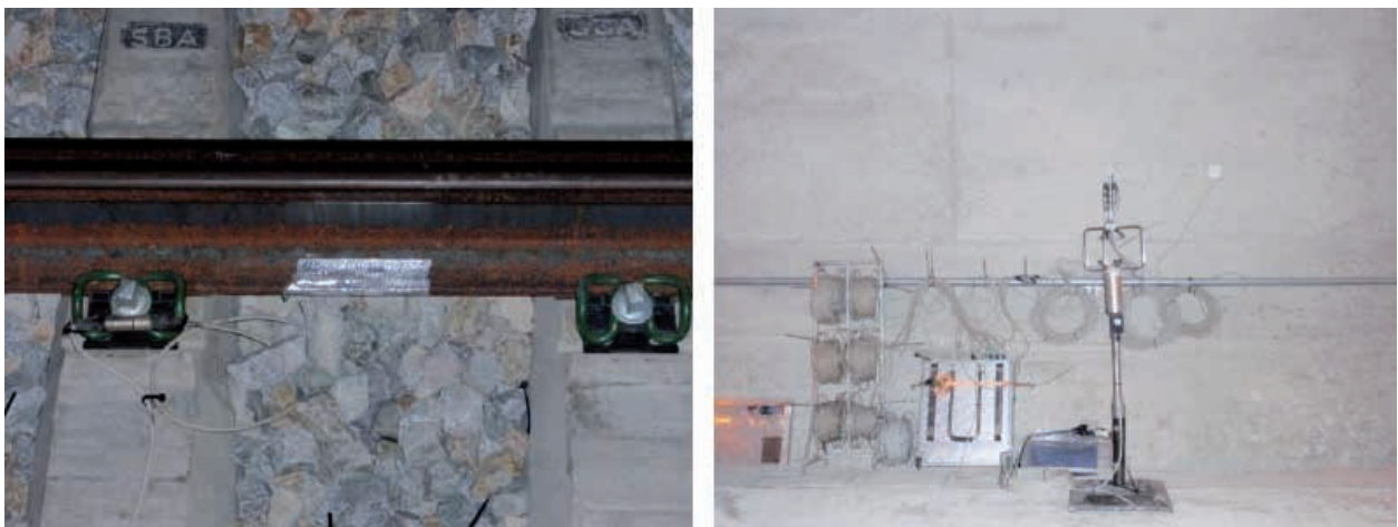
Figure 9. Instrumentation set in La Cabrera Tunnel
